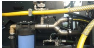
One of our features are the efficient and clean installation of the booster line (stainless steel) with a huge, final water filter and a filter inlay of 1 or 0.45 micron
